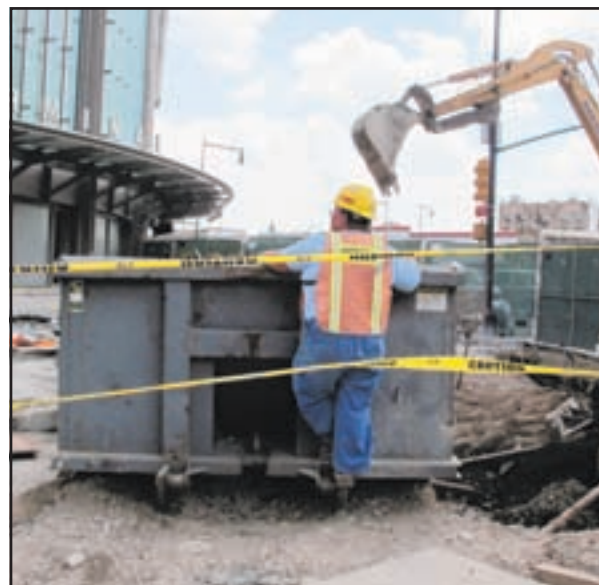
ROCKS GONE: Construction workers ripped out the giant granite bollards that blocked pedestrian walkways in front of Atlantic Terminal since a 2010 renovation.
