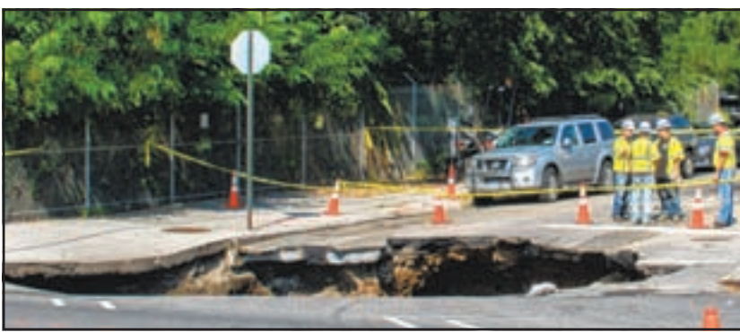
NOW THAT'S A HOLE!: Workers are still fixing the massive sinkhole that swallowed the corner of 64th Street and Fifth Avenue in August. Photo by Georgine Benvenuto
