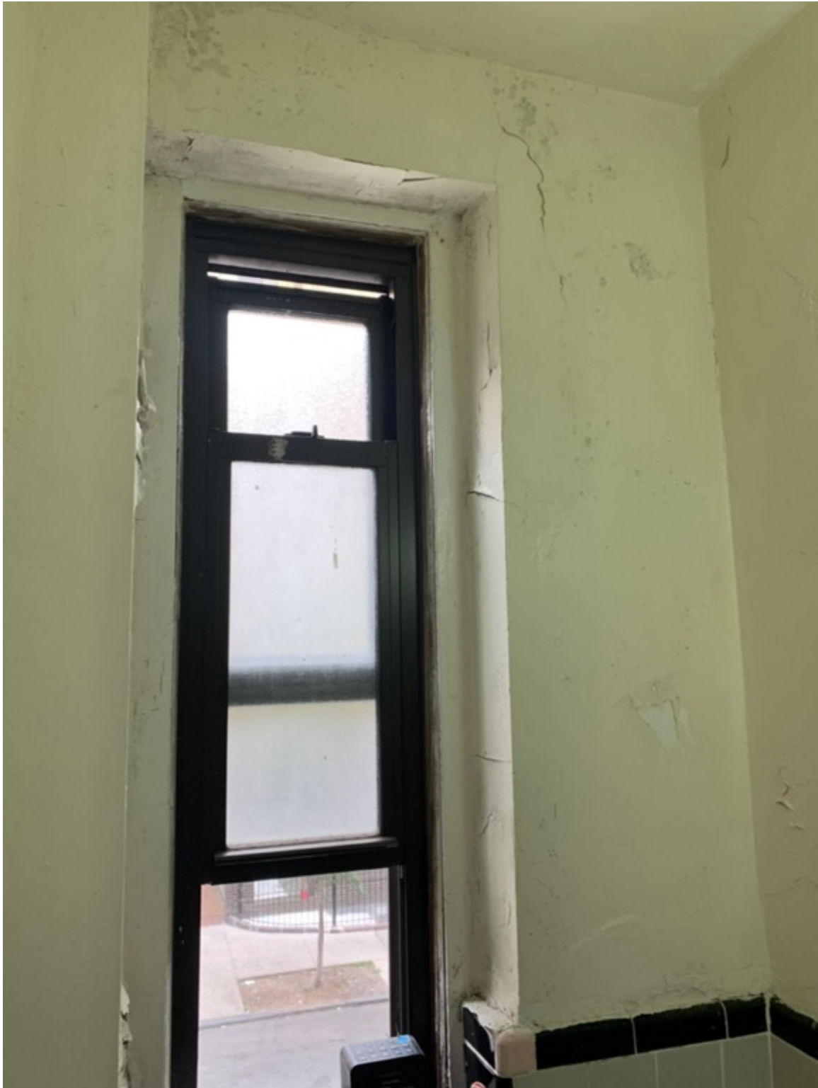
Mold growth and water damaged in the 2C bathroom
