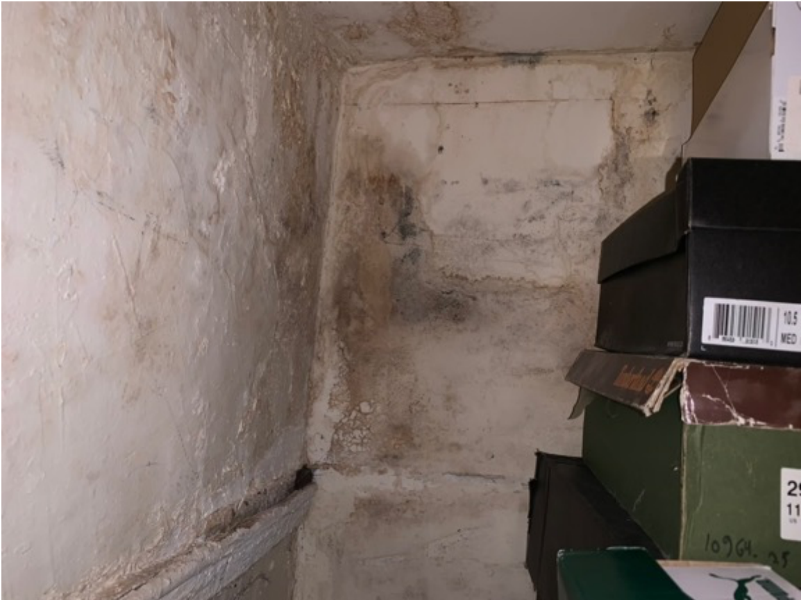
Moldy bedroom closet in 2C
