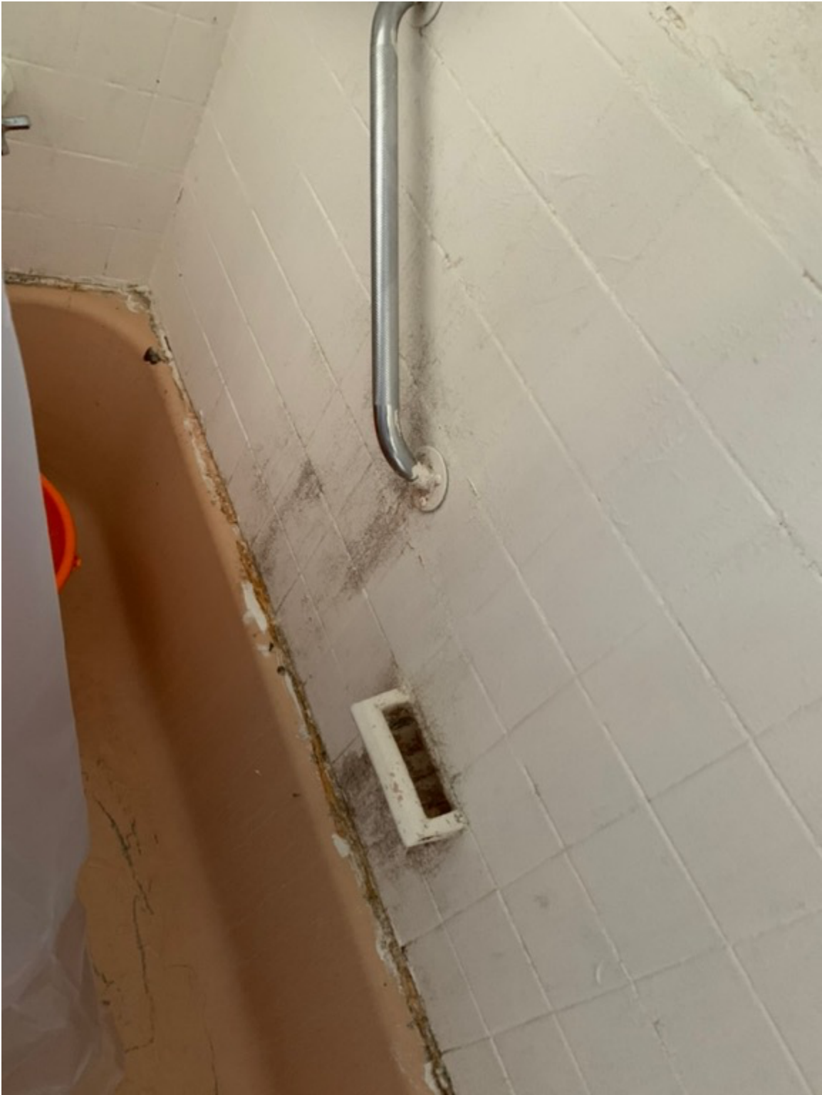
visible mold around the tub in 5B bathroom
