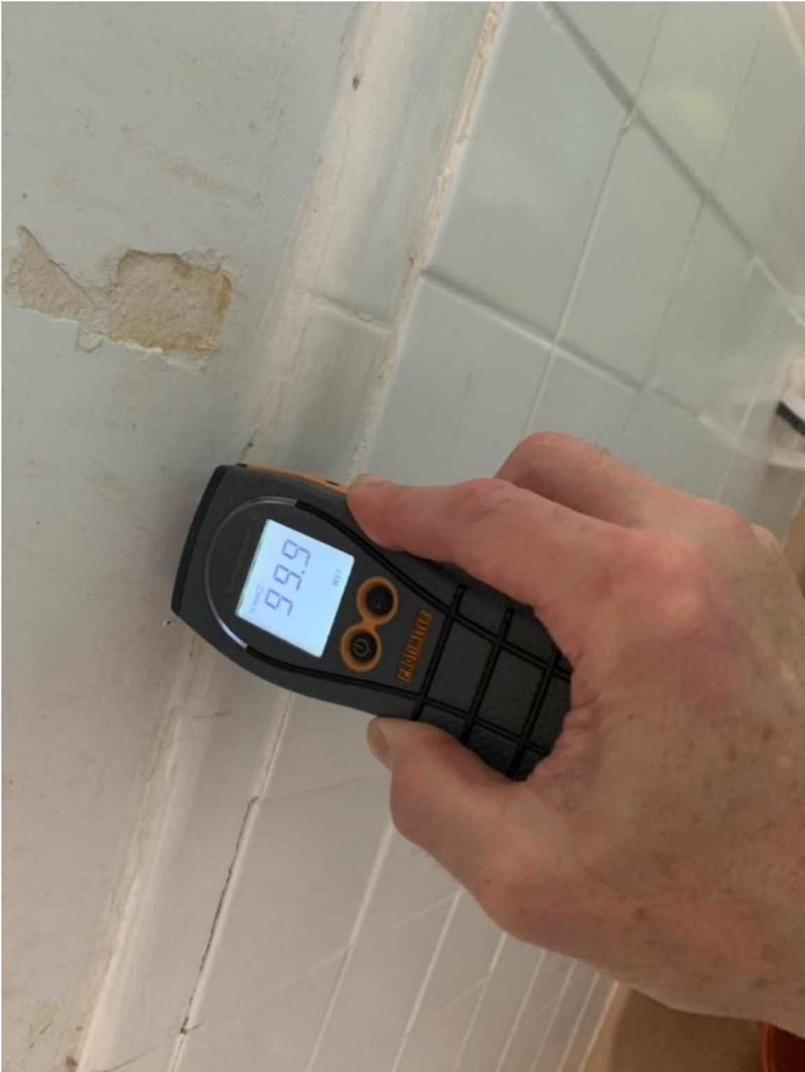
apartment 6B – the walls are soaked around the tub
