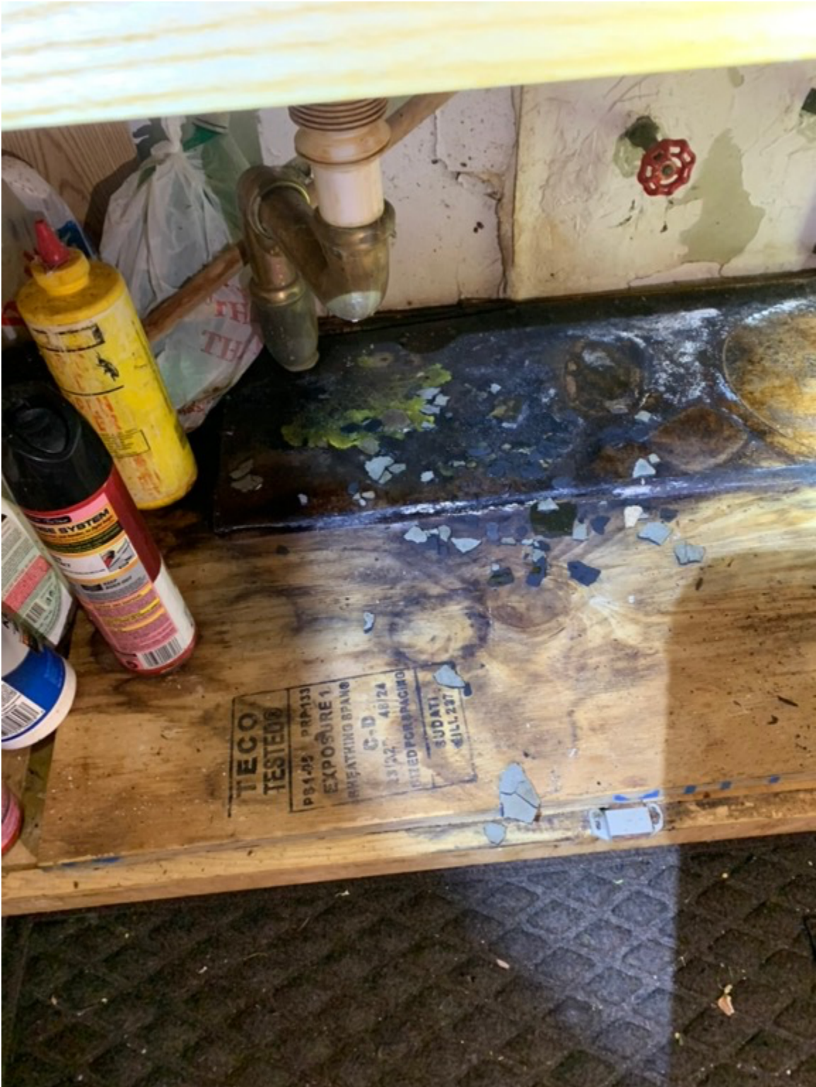
The sink in the kitchen in 6B is water-damaged and moldy
