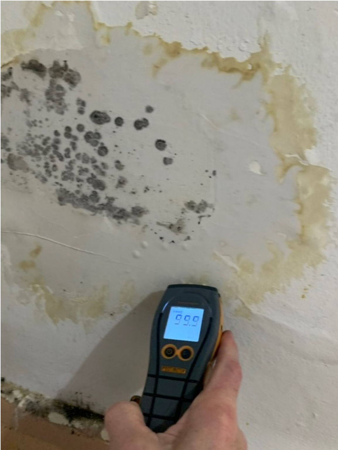
3A bathroom walls are soaked and saturated with sewage
