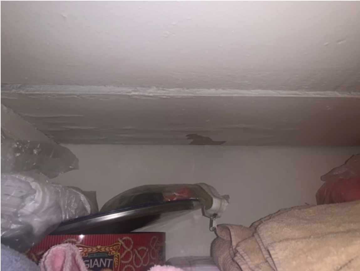
damage to the bedroom closet 3C
