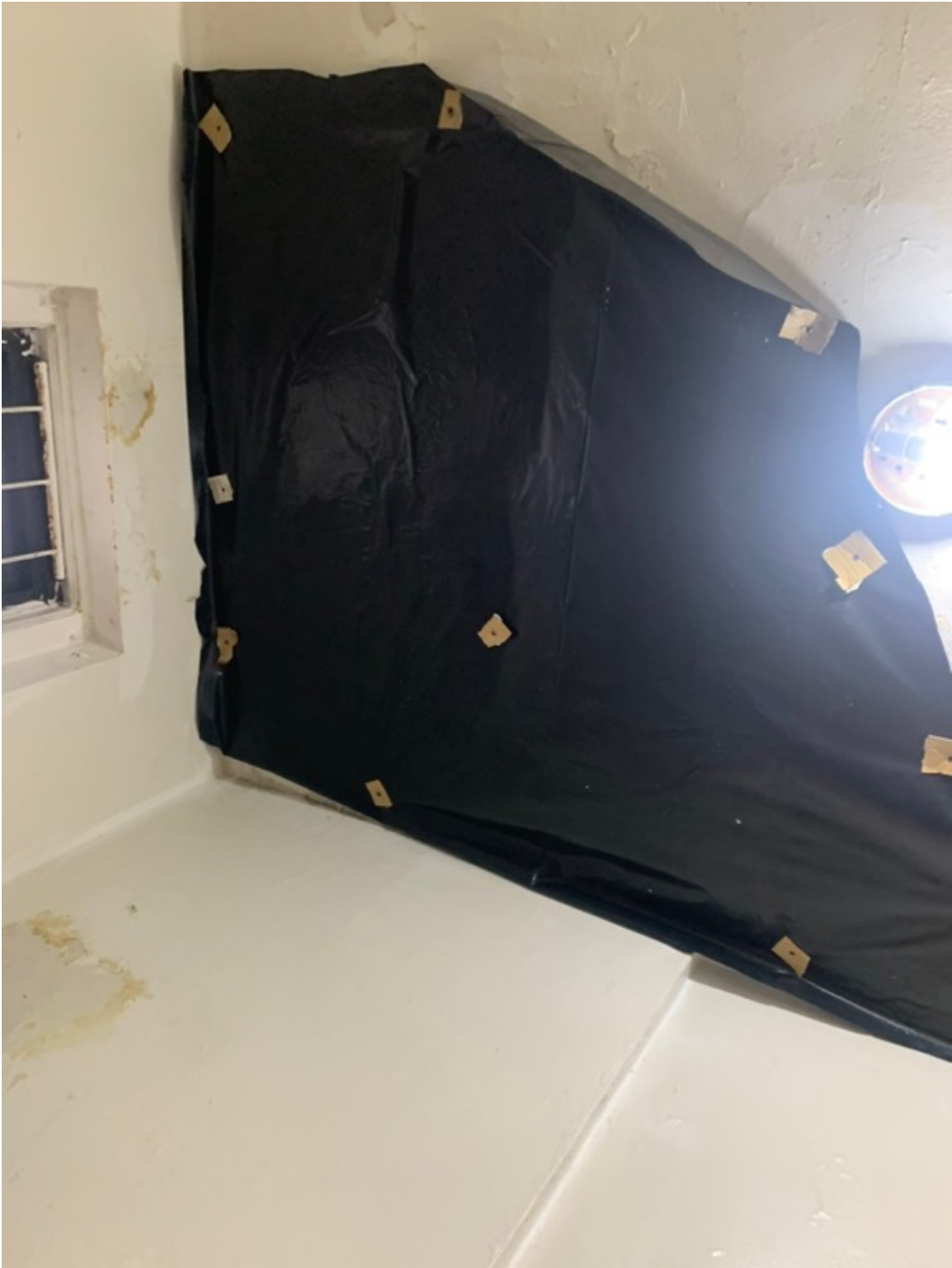
bathroom ceiling in 3A – sewage is leaking
