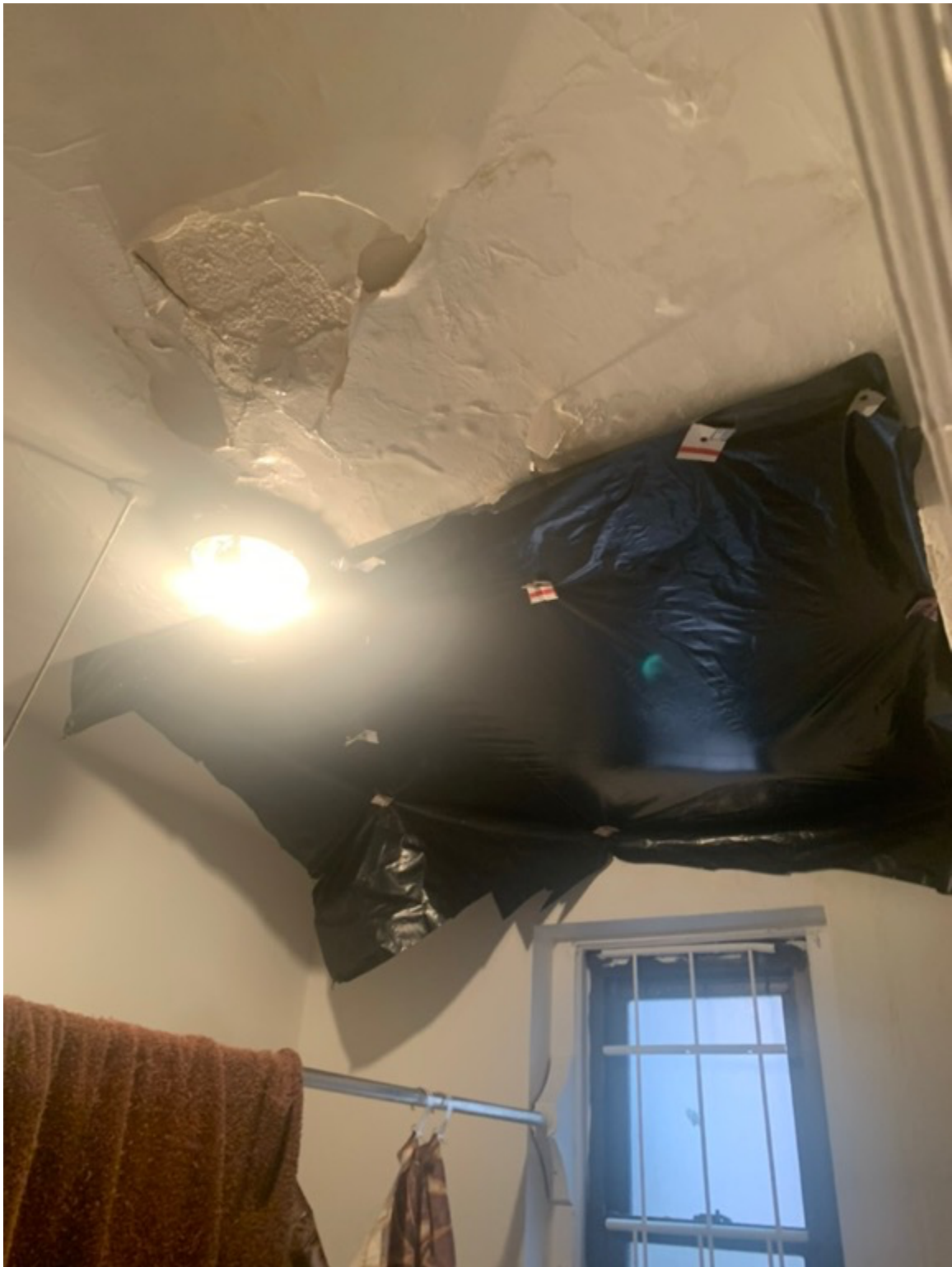
sewage leak in 4A bathroom
