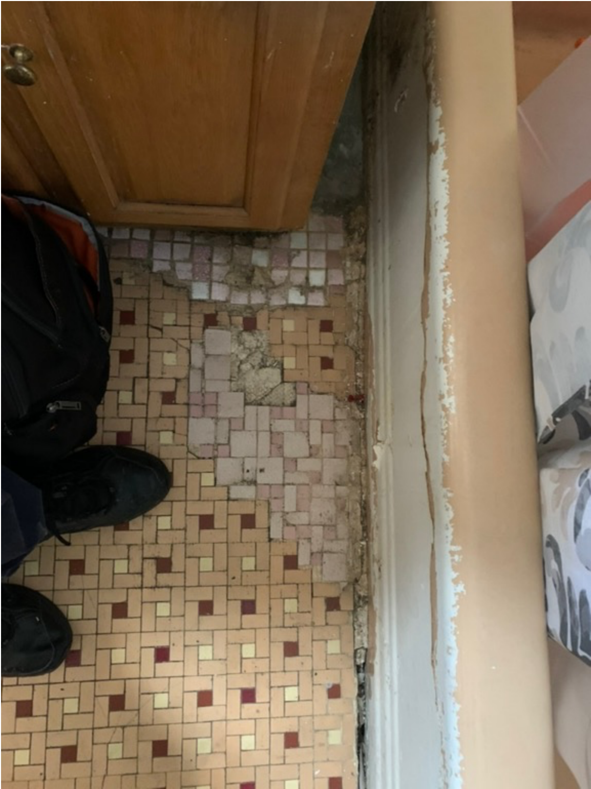
The damaged floor in the 5B bathroom
