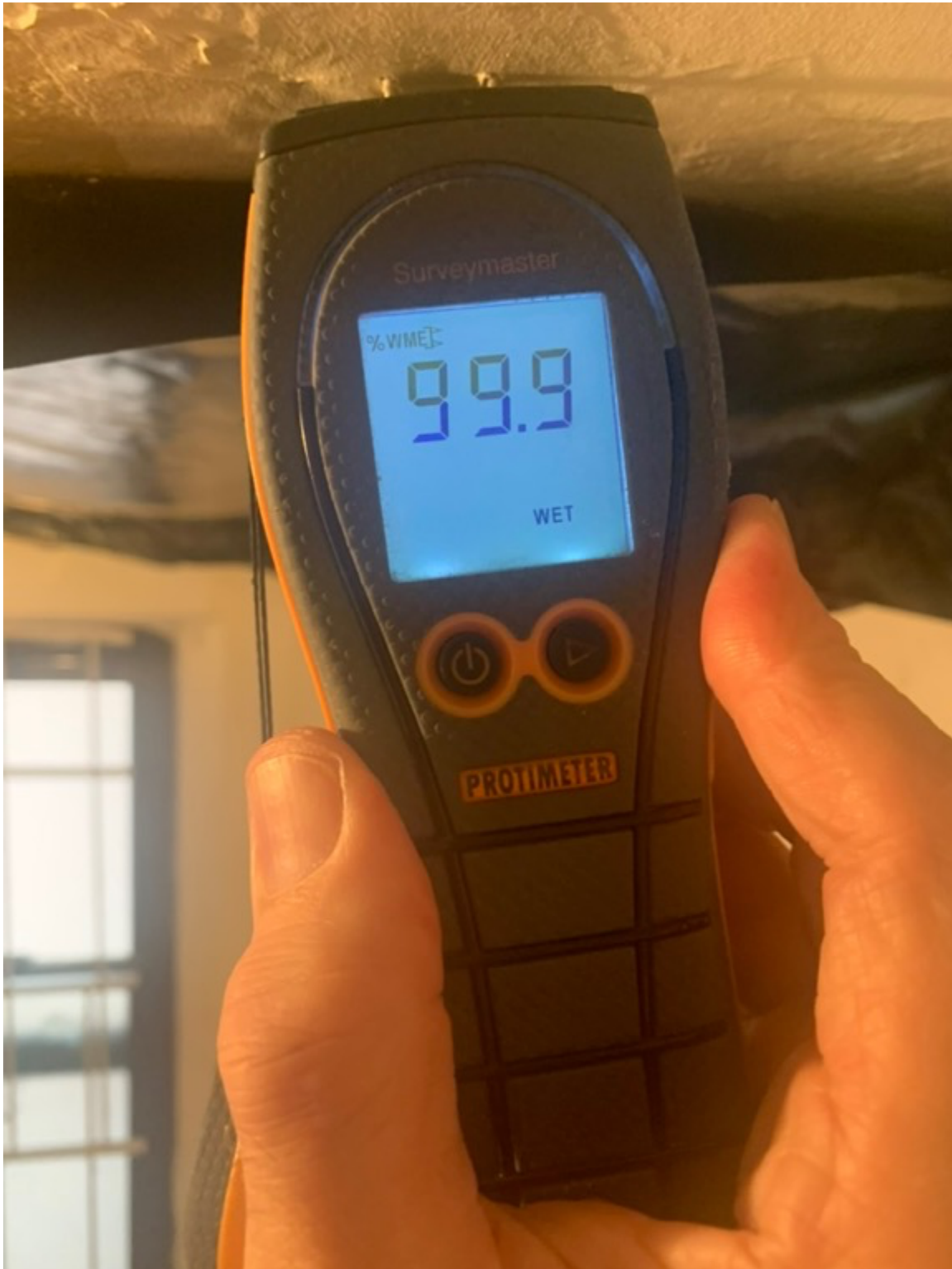
soaked bathroom ceiling 4A
