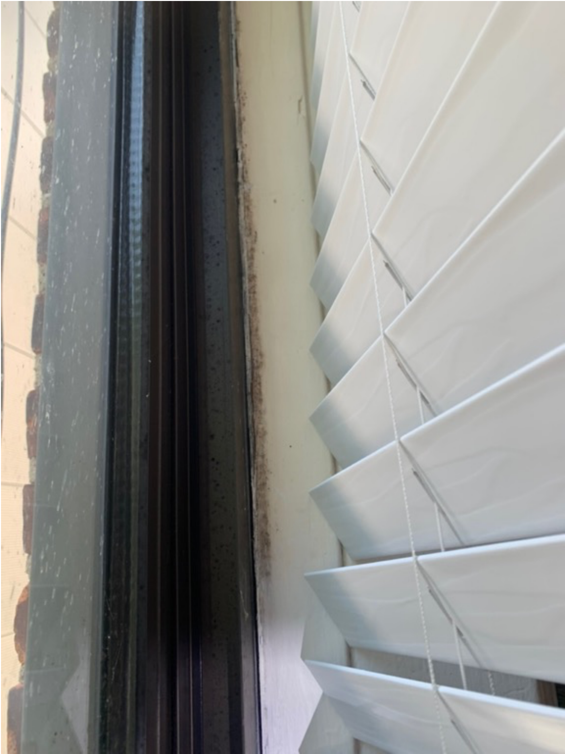
Mold growth around the windows in 5B
