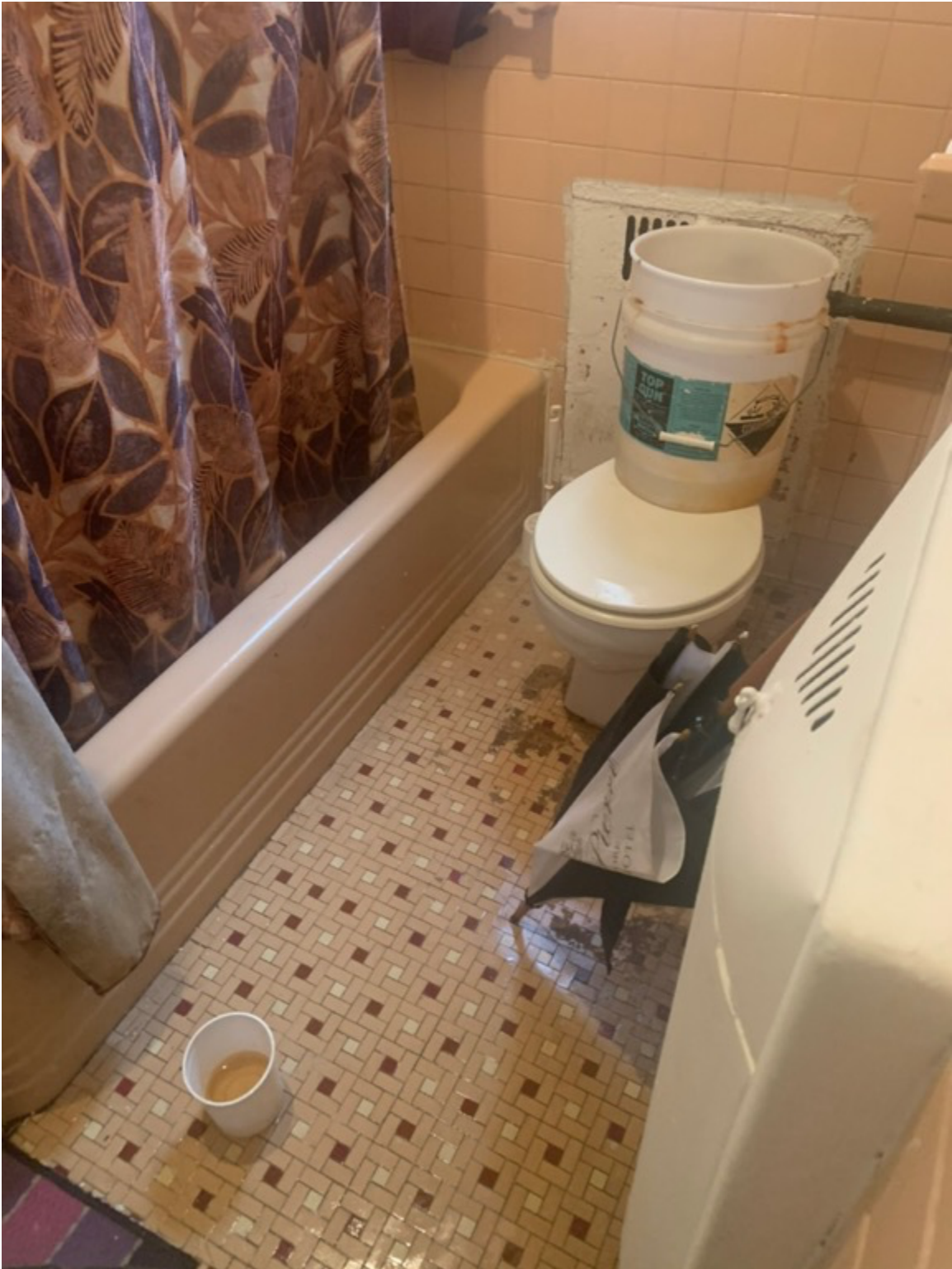
the floor is wet from dripping sewage in apartment 4A bathroom
