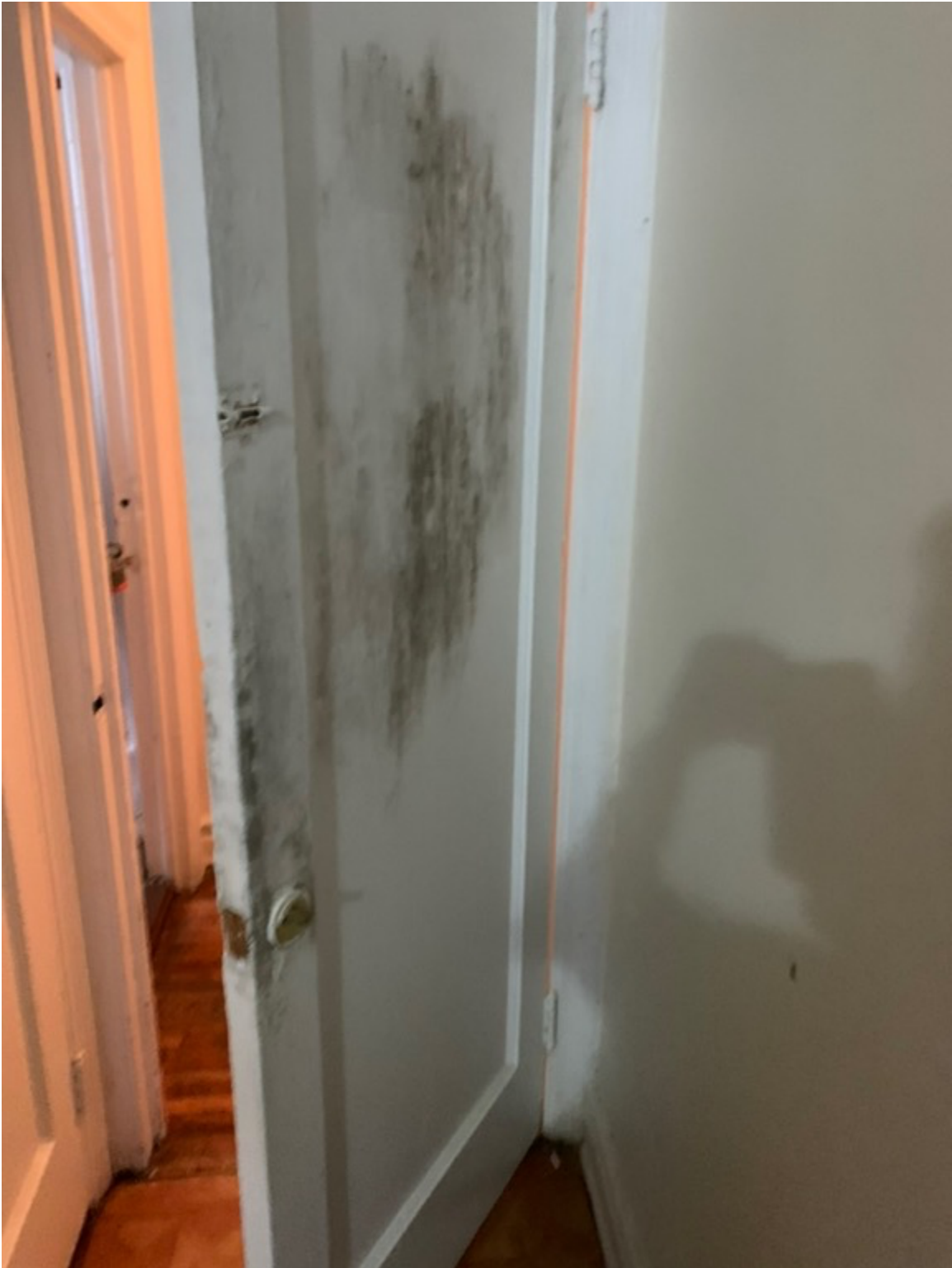
visible mold on the bedroom door in 5B
