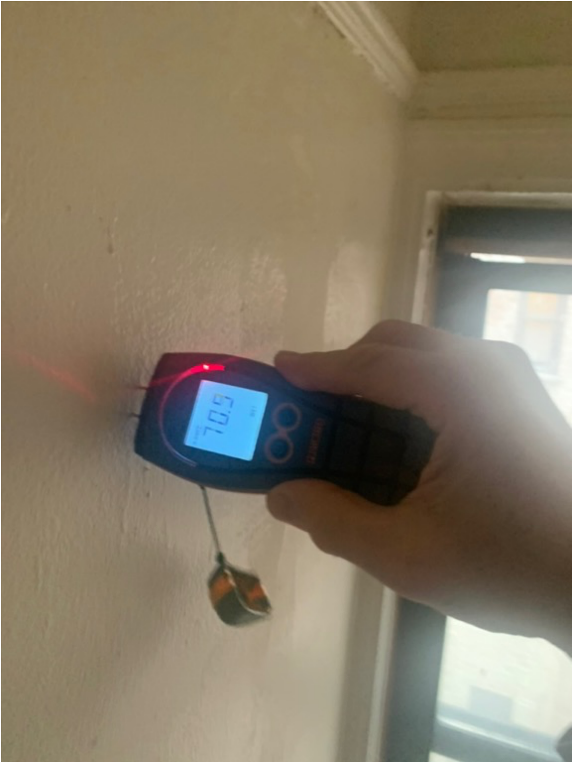
moisture in the hallway wall in 4A long wall shared with the bathroom
