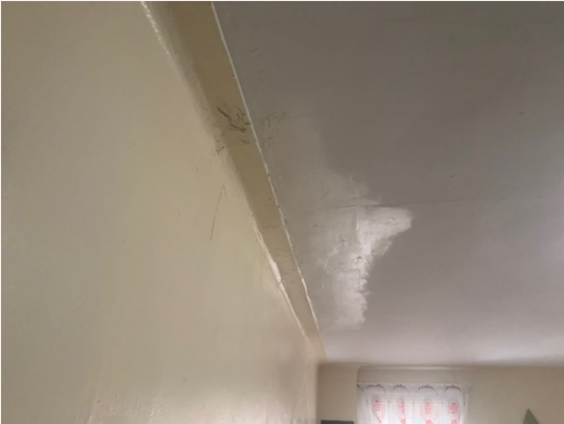
damage and moldy plaster in the living room of 3C
