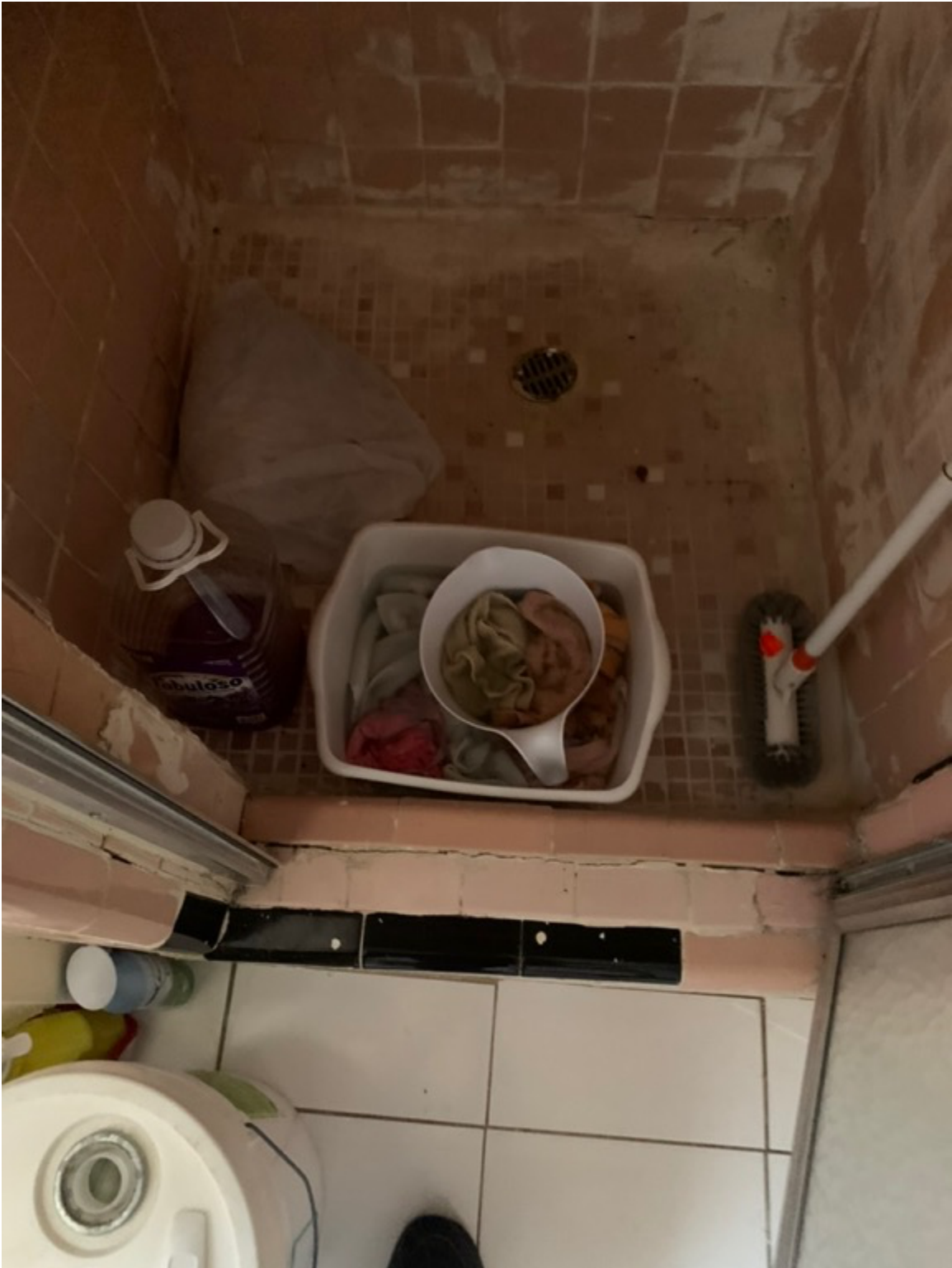
The shower in 5F is in poor condition and cant be used
