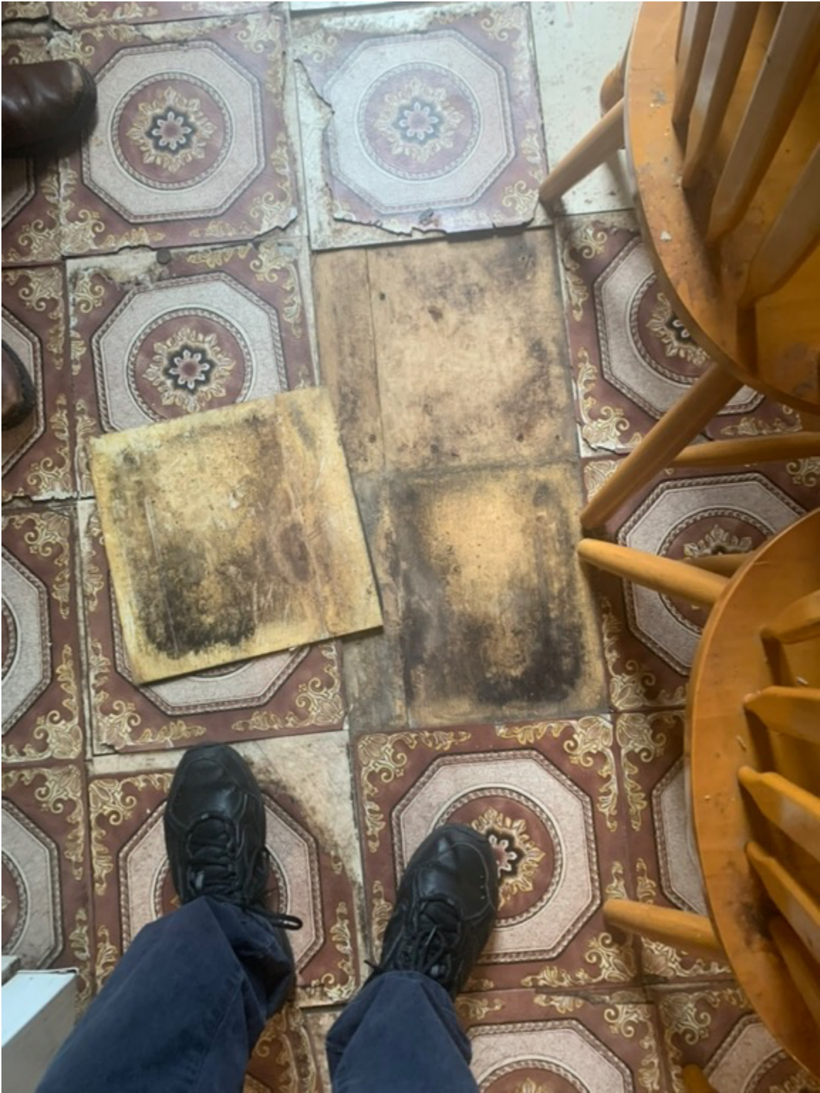
Moldy floor in the kitchen in 4A
