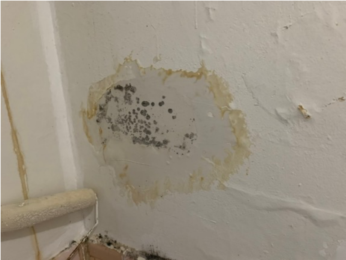
visible mold in the bathroom of 3A – there is an active sewage leak
