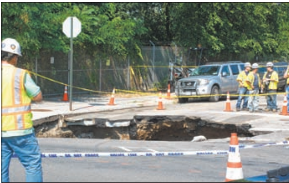
FIXING A HOLE: Utility and city workers examine the yawning sinkhole that suddenly opened at the corner of Fifth Avenue and 64th Street in Sunset Park on Aug. 4 – but locals say they saw it coming.
