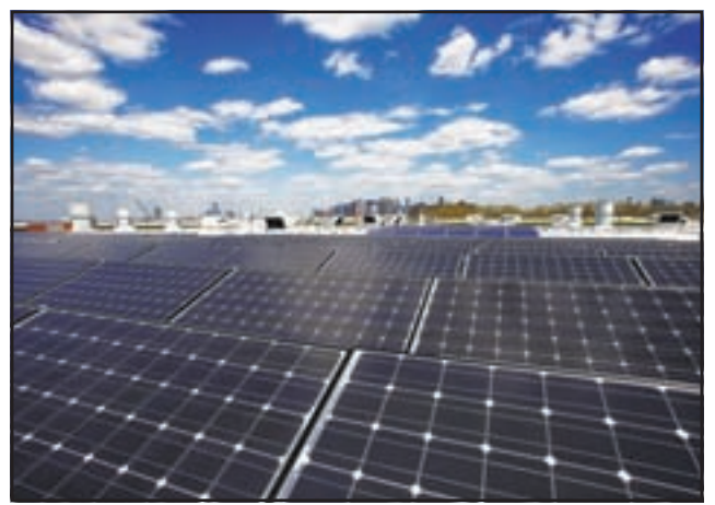
EVERYBODY LOVES RAYS, MAN: Solar panels on the roof of Ikea in Red Hook. Associated Press / Mark Lennihan
